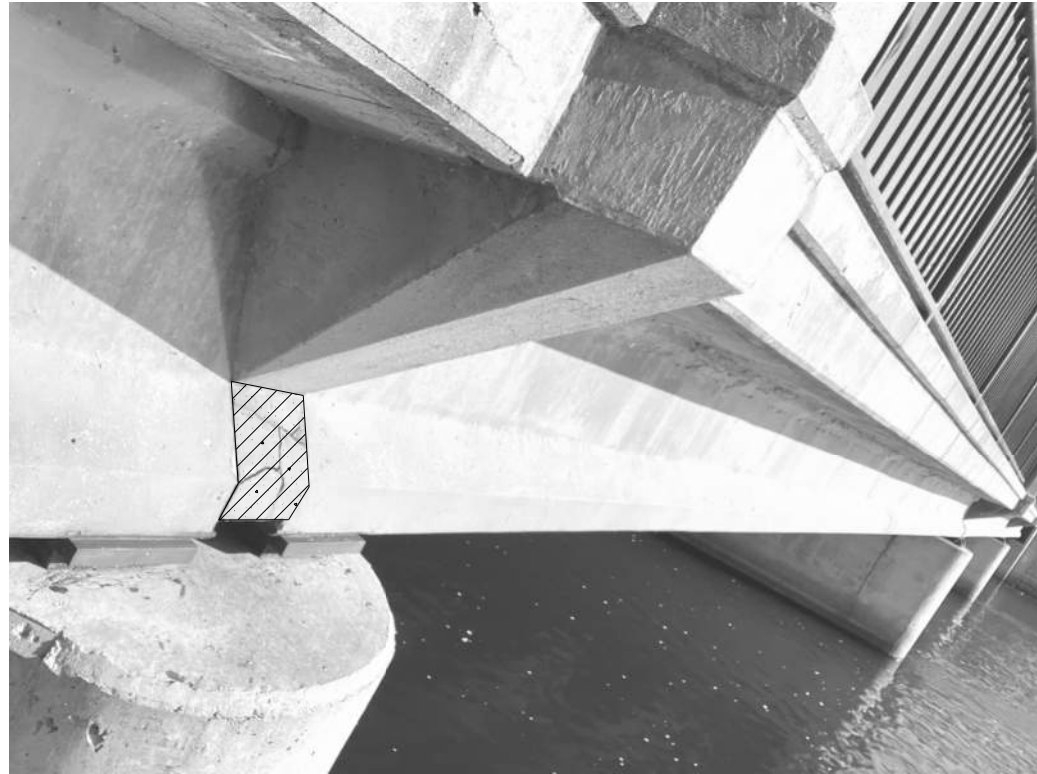
EXAMPLE PIER DIAPHRAGM SOUTH END WITH DETERIORATION (For information only)
