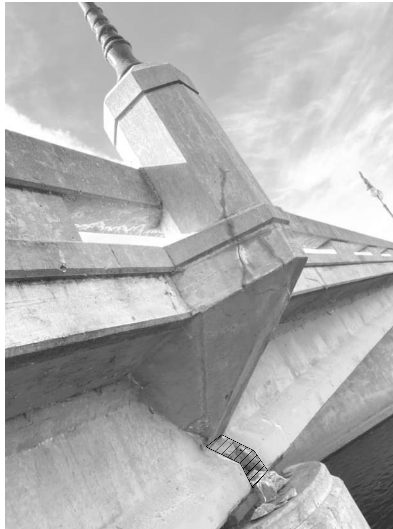
EXAMPLE PIER DIAPHRAGM NORTH END WITH DETERIORATION (For information only)
