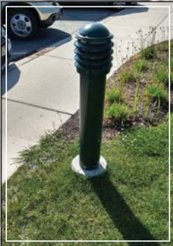
Walkway Lighting Bollard with Integrated Power Source
